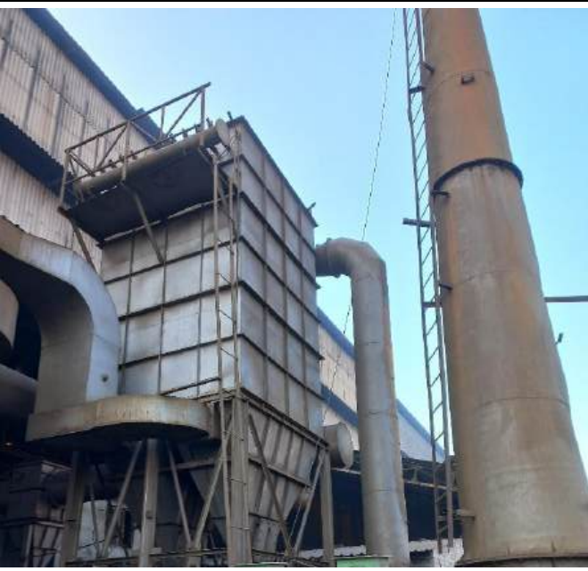
AIR POLLUTION CONTRLL (APC) SYSTEMS
